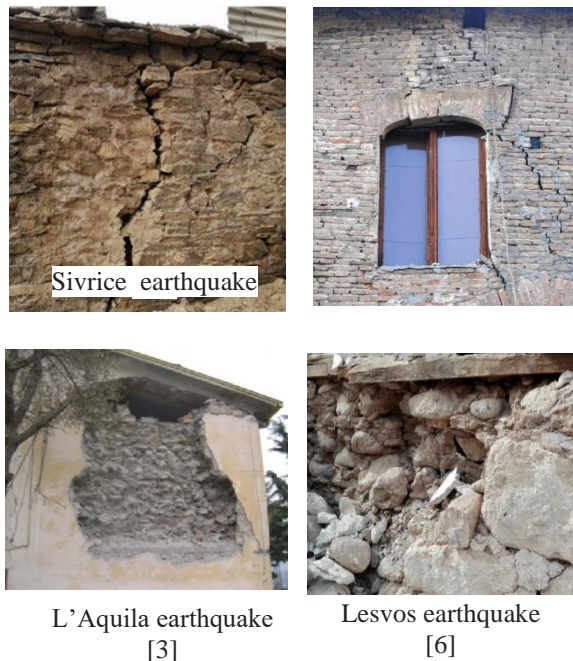
Figure 1. Damage situations of masonry structures
