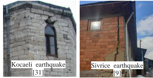
Figure 1. Continue Damage situations of masonry structures
